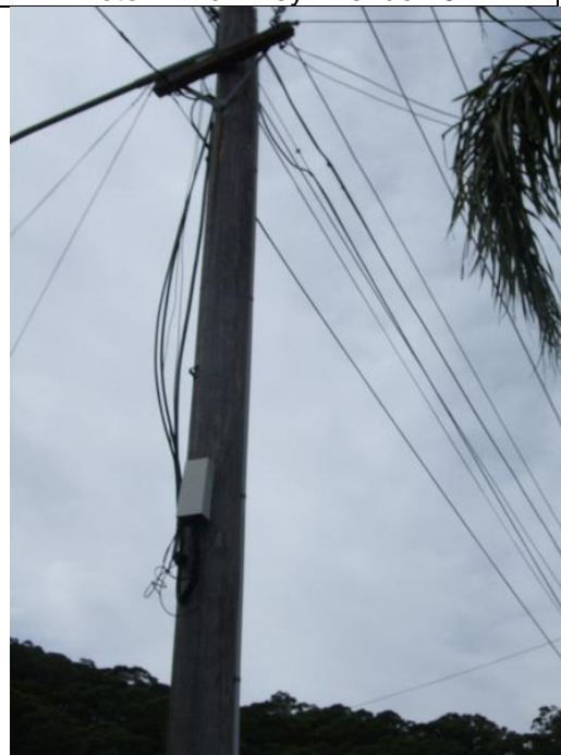
Photo 4: The fragility of aerial copper telephone cables
